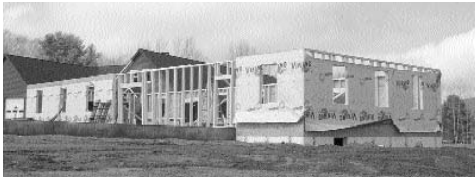
The new Thomas Miller Jackson Building, currently under construction, will provide space for the Studio Fellowship Program.
